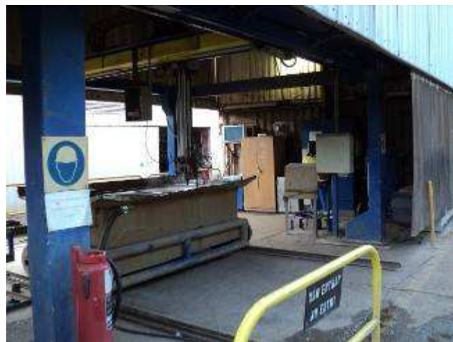
Figure 5: Now we have made the service because too much sand on the roller guide and the racks was driving, causing restless movements.
