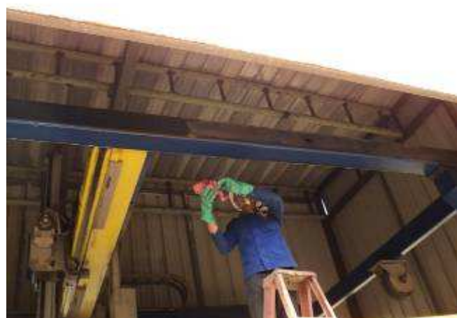
Figure 6: According to the provisions in the camp, the scaffolders must stand a scaffold because over 1.8 meters allowed to work from the ground only with scaffolding. If a scaffolders comes and the Machine is urgently needed, selects alternatives.
