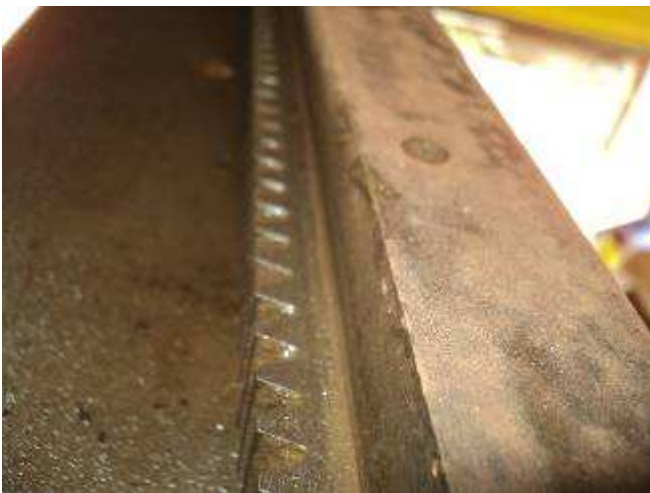
Figure 8: Here we see how the racks and guides look. Also, rust and sand cause irregular operation.
