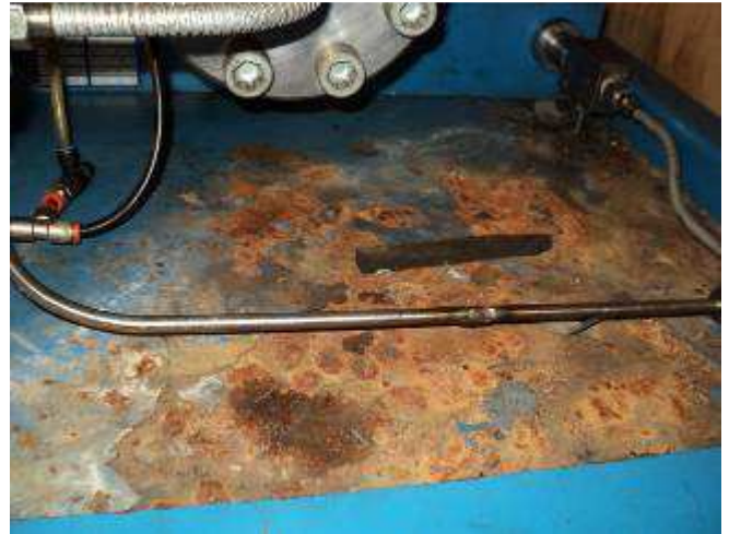
Figure 11: This is also a defective pipe was welded. Through these tubes but goes beyond 3000 bar pressure, so we have organized new pipes from Switzerland, so that they can be replaced. Is not without danger.
