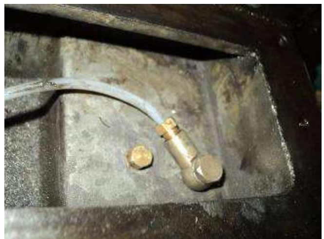
Figure 32: There were drilled new holes which supply the guides with oil.
