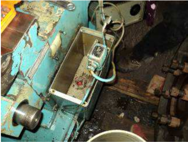
Figure 23. But the bed track lubrication container was cleaned inside. It was like many times before, a lot of dirt in the tank.
