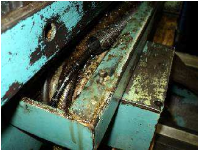
Figure 28. When a trailing cable cover is opened, it looks like this. Dirty and waiting for maintenance.
