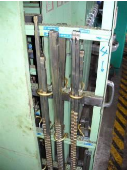
Figure 10: protected too, with grease
