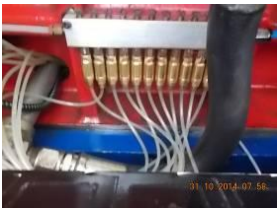
Figure 13) The old, existing lubrication system has no pressure control, thus
