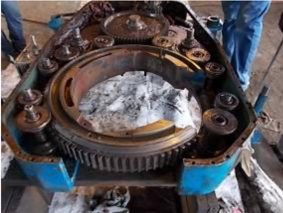
Figure 66) The transmission from the inside looks very dirty.
