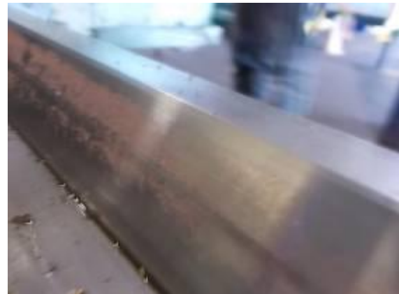
Figure 73) The rust is a big problem in Angola.
