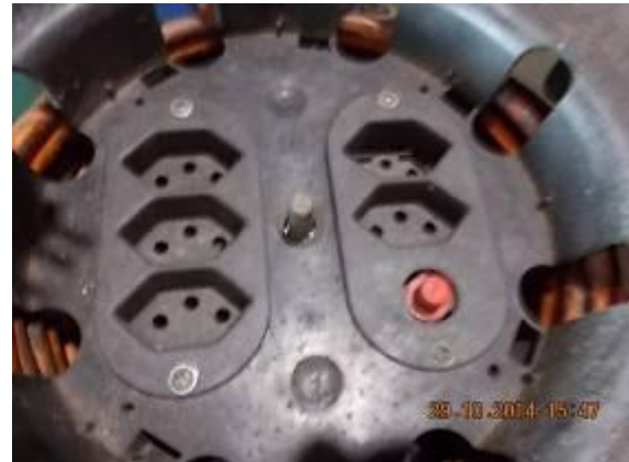
Picture 48b) Swiss cable reels for 10 Amp. Not 16!
