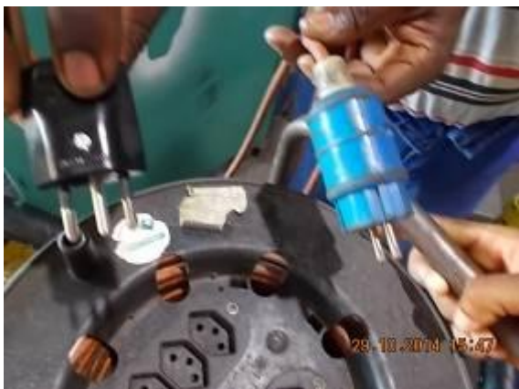
Picture 48a) Many cables roles in Algoa have the Swiss plug. These are designed for 10 amp. Now the plugs are cut off in many new and mounted.
