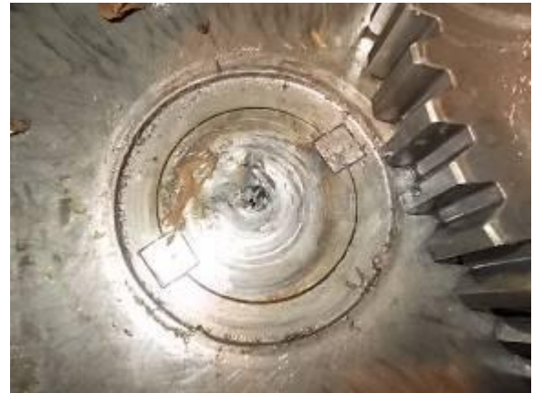
Figure 63) Some damaged areas.
