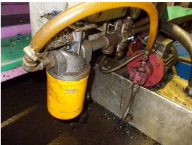
P13: At the Gornati: With all CNC machines of the WIAP, it has 10 micron filter. Outside with a signal switch, so that the dirt in the oil can be intercepted. Each gear of the machine with the filters, can after 10 years of gearbox cover be lifted. It does not have any traces of dirt.
