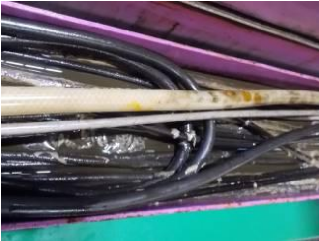
P22: A water hose rupture in the energy supply was a big mess.
