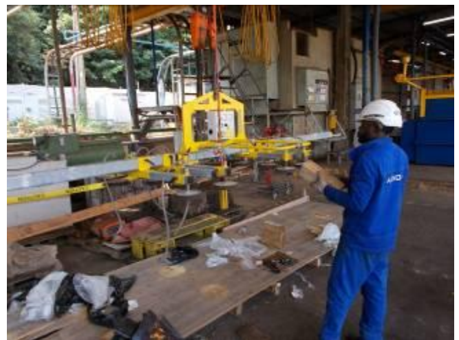
P61: The wooden floor is broken through. The suction cups standing on the ground. That was not the goal of the package.
