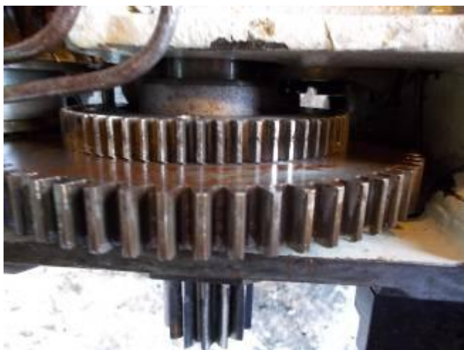
P37: The defective wheel, the smaller, the more teeth are broken. Was welded and repaired. Unfortunately not good enough. The old module was chosen wrong because the break anything so deformed that it could not be determined correctly. When the gear was worn with the dividing head, teeth were once with too little, then again with too great a distance.
